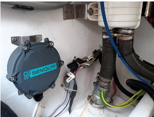
Figure 1 - ORB-X1-G Installed in the Engine Bay
