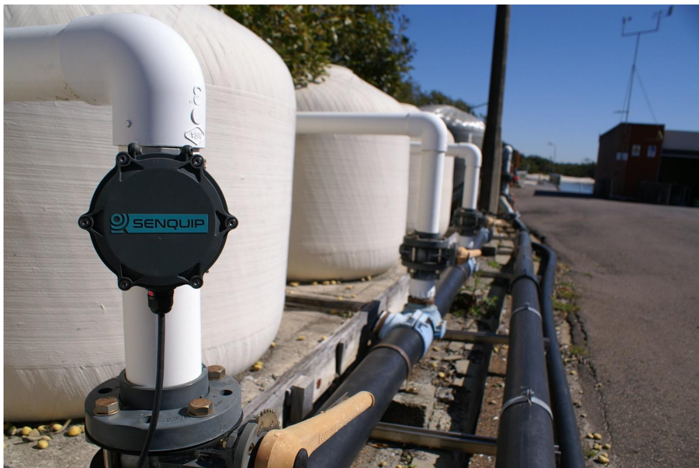
Figure 3 - Battery Powered ORB-X1 Monitoring Filter Pressure
