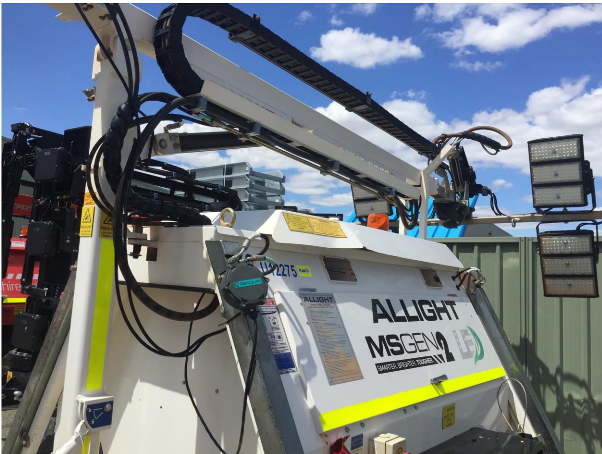
Figure 13 - Typical Lighting Tower with Serial Communications
