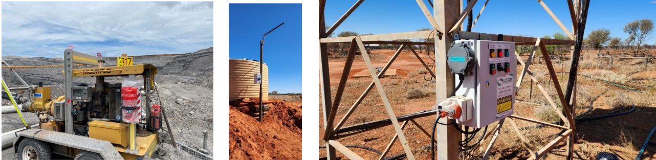
Figure 1 - Selection of Pumps Controlled and Monitored by Senquip Devices
